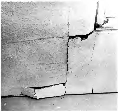
Photo 11. Van Gogh Street Elementary School. Underside of roof overhang damaged above ground cracks.
